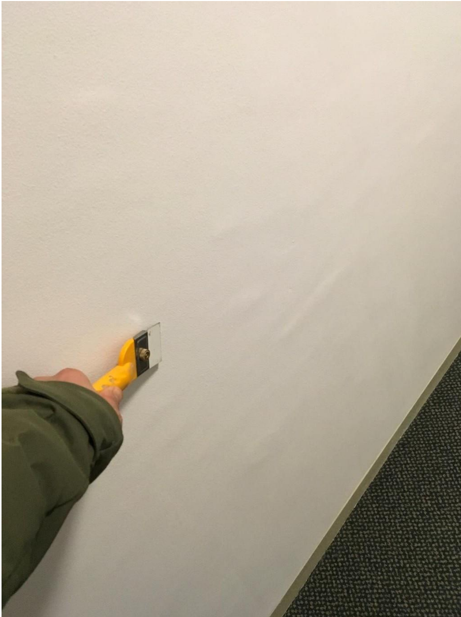
Fig 6, Walls are not smooth and even
