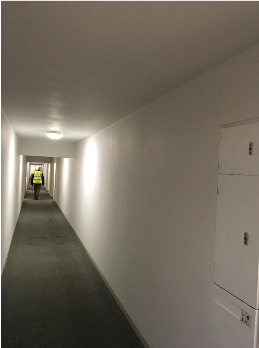
Fig 5, streaky finish on ceiling when viewed from angle however when viewed face on no patchy/streaky effect was observed
